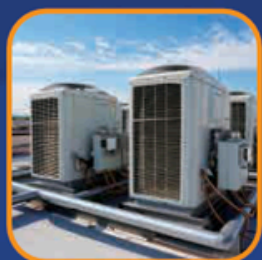
Air conditioning equipment
