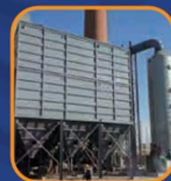
Air purification equipment
